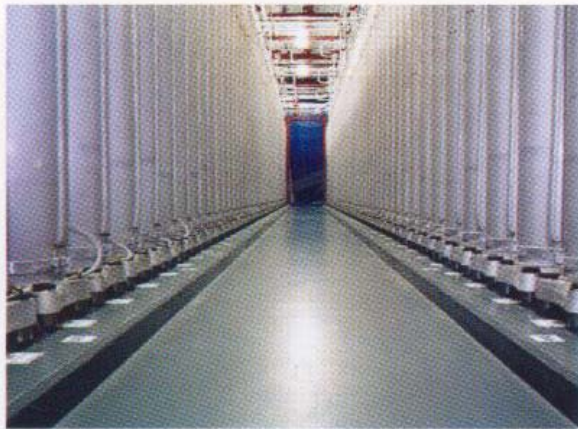
Cascade hall at Urenco Plant, Capenhurst, UK
